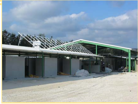
The framework for our solar panels is in place - our main source of power will be solar
